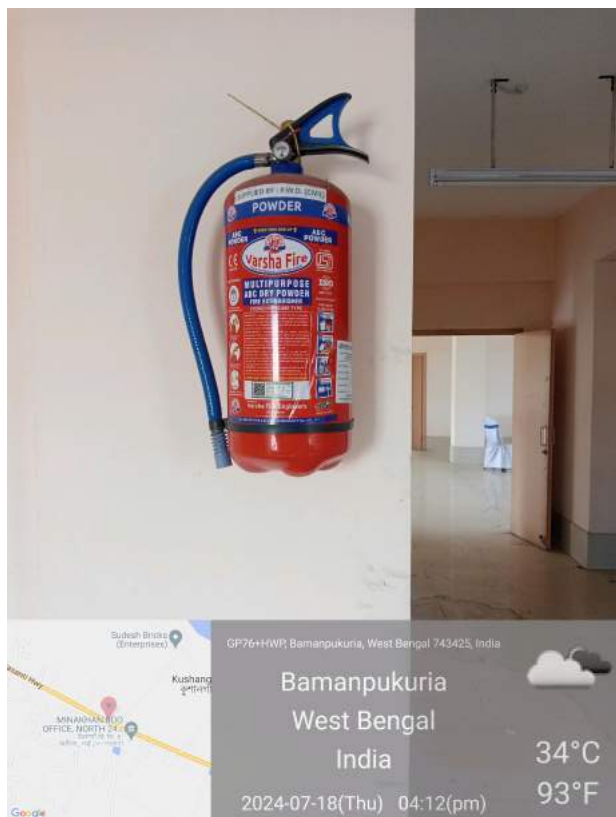
Fire Extinguisher System
